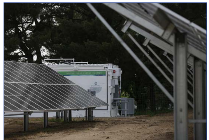
Battery storage with solar arrays
