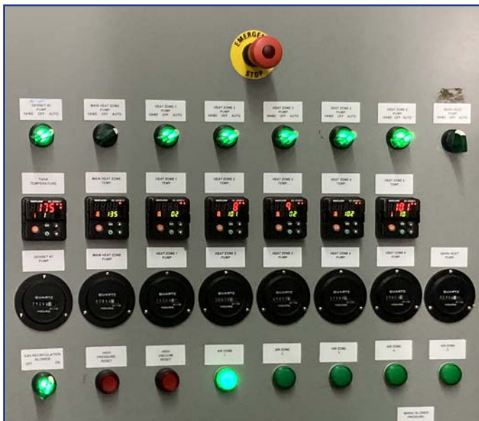
Digester heat pump monitoring
